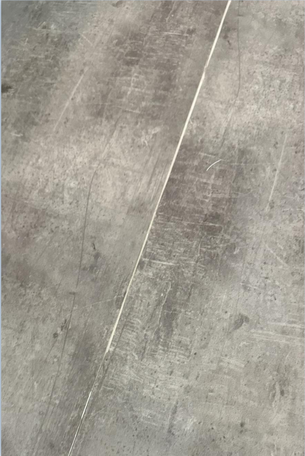
Before – Gap Visible
